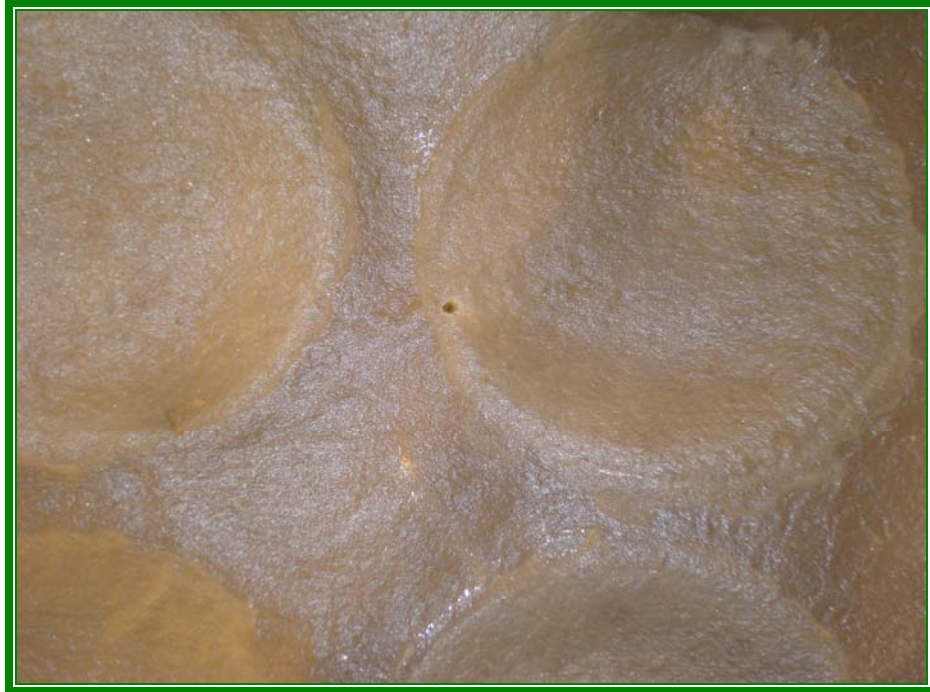
Termite penetration through Sopraseal LM 200 T (Top Side View)
